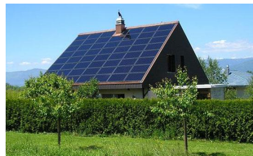
Example of a Solar Conversion System, Structure-mounted
