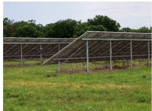
Example of a Solar Conversion System, Ground-mounted
