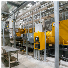
Power and Electric
