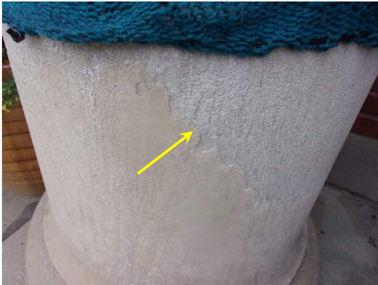
Figure 17: detail of spalling at column.
