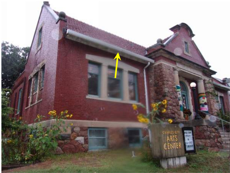
Figure 19: leak at existing gutter and downspout.
