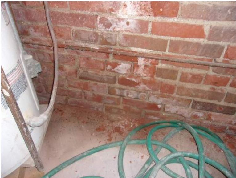
Figure 10: deteriorated masonry at south corner.
