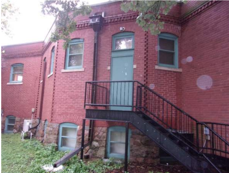
Figure 23: collection box, downspout, and discharge.
