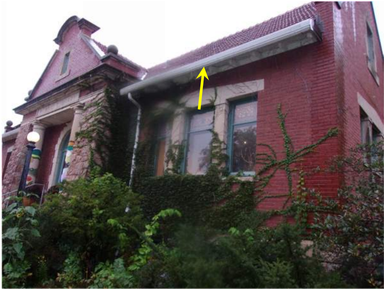
Figure 21: leak at existing gutter and downspout.
