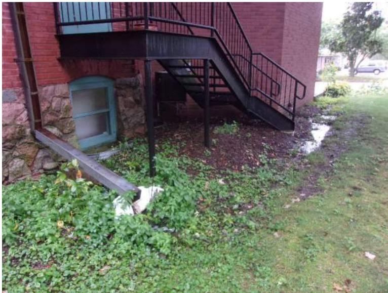
Figure 24: discharge and water migration towards storm drain.
