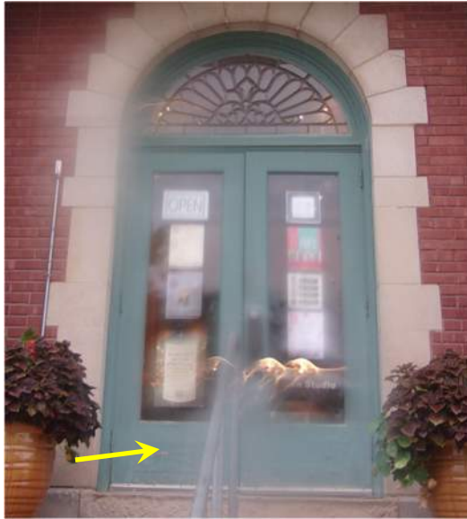
Figure 18: finishes deterioration at entrance doors.
