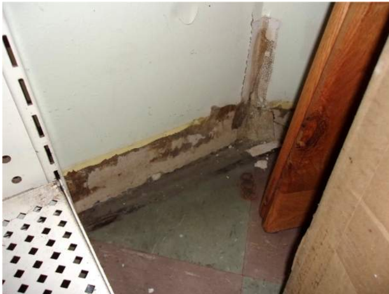
Figure 5: Painting Studio, base of wall showing prior water damage.
