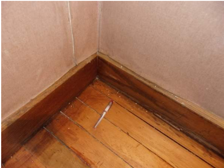
Figure 15: wood floor landing and seams at the wall covering.
